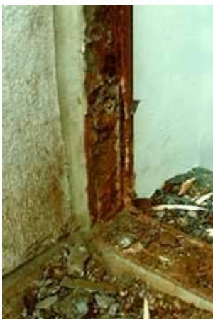
A severely deteriorated frame, such as this, can be replaced in kind. Photo: Henry Chambers, AIA.
