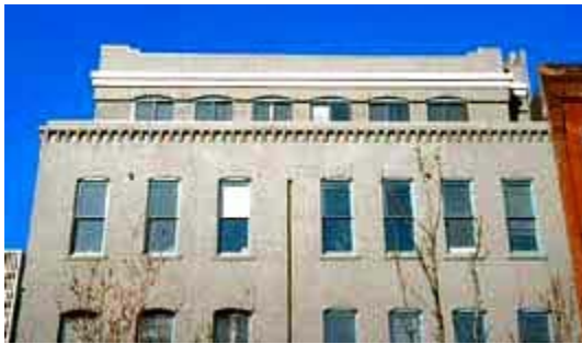
This highly visible new rooftop addition appears to be part of the historic building because of its replicative design and historicized detailing, such as the arched windows. This approach does not meet the Standards for Rehabilitation. Photo: NPS files.
