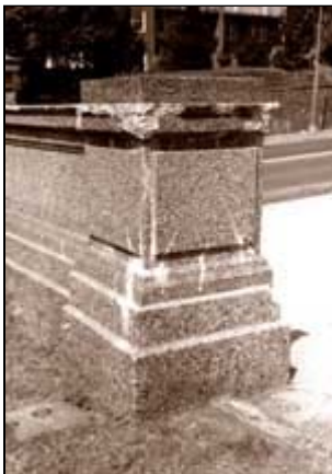
This reinforced concrete pier at Meridian Hill, Washington, DC, has lost much of its projecting molding partly from accidental impact and partly from spalling induced by freeze-thaw action. Photo: NPS files.
