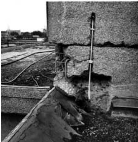
Prior to repairs of the Unity Temple, Oak Park, Illinois (1906), spalled concrete was most noticeable at locations of concentrated rebars. Deteriorated concrete, the 1960s stucco finish, and corrosion were removed by grit blasting. Photo: Robert Bell.
