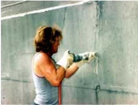
At the Virginia Heating Plant, Arlington, Virginia (1941), narrow cracks needed to be widened to receive concrete patches. Photo: NPS files.
