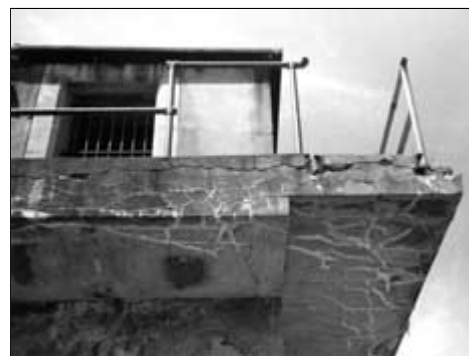
This 1904 reinforced concrete tower (Battery Commander's Station, Fort Washington, Maryland) is showing serious deterioration. Water has penetrated the slab, causing freeze-thaw spalling around the posts and corrosion of the reinforcing bars. Photo: NPS files.
