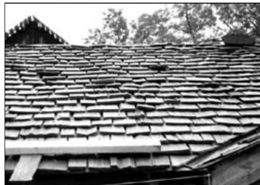
These commercially available roofing products with rustic split faces are not appropriate for historic preservation projects. Photo: NPS files.
