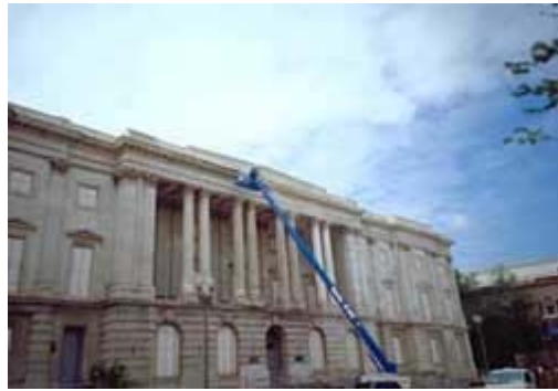
Low-to-medium-pressure steam (hot-pressurized water washing) is a gentle method of softening heavy soiling deposits and cleaning historic marble. Photo: NPS files.
