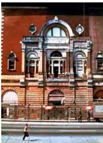
Ninety years of accumulated dirt and pollutants are being removed from this historic theater using an appropriate chemical cleaner, applied in stages. Photo: Richard Wagner, AIA.
