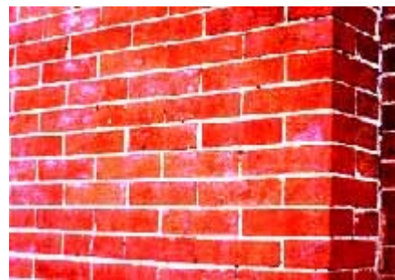
Improper cleaning methods may have been responsible for the formation of efflorescence on this brick. Photo: NPS files.
