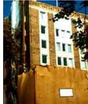
The lower floors of this historic brick and architectural terra-cotta building have been covered during chemical cleaning to protect pedestrians and vehicular traffic from potentially harmful overspray. Photo: NPS files.
