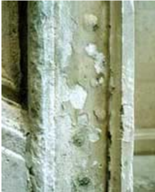
This clear coating has failed and is pulling off pieces of the stone as it peels. Photo: NPS files
