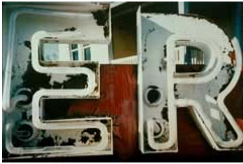
These tubes in this amusement park's sign were broken and the surrounding "metal cans" needed work also. See below. Photo: Stan Fowler.
