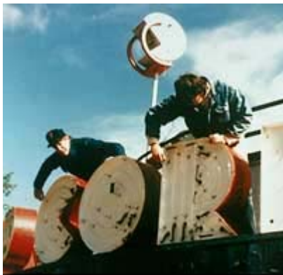
Neon fabricators are installing the new tubing in the repaired and remounted cans. Photo: Larry Kanter.
