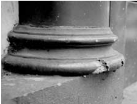
This lightweight fiberglass column at street level sustained damage from impact within a few years of installation. Photo: Building Conservation Associates.
