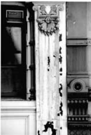
On this building, a strong alkaline paint remover was used, and apparently was not adequately rinsed or neutralized. Over a period of months, the newly applied paint began to peel and streaks of rust appeared on the iron. Photo: Kim Lovejoy.
