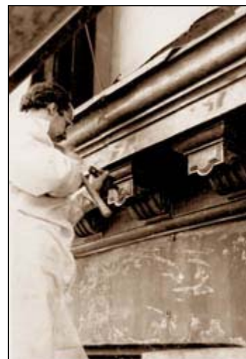
Where chemical paint stripping is involved, careful planning of the sequence of work and inspection by an architect or
