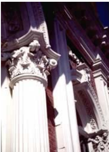
Fiberglass columns and aluminum capitals were installed to replicate the ornamental features on the east facade of the New Market Theater in Portland, Oregon.
