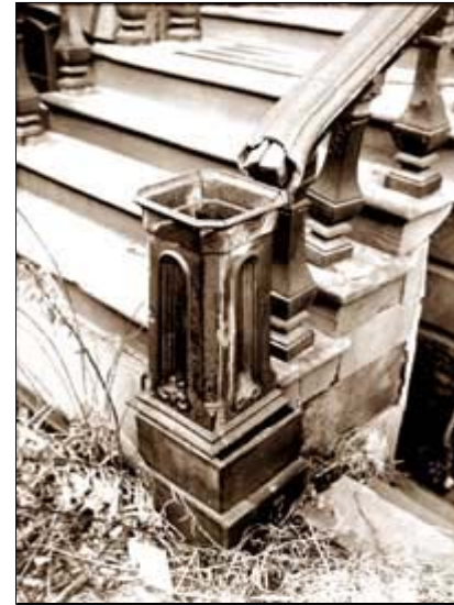
In an effort to repair the stair railing, concrete was poured around the wood spacer inside the railing ceiling. Water penetrated the railing and reacted with the concrete to accelerate the corrosion of the iron. Photo: John G. Waite.
