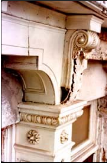
Structural crack, gaps at joints between components, and a large opening where part of the console bracket is missing are the problems evident in this cast-iron assembly. Photo: Ford, Powell & Carson.
