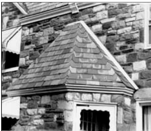
The white blotches on these Pennsylvania Soft-Vein slates indicate areas where gypsum is leaching out onto the surfaces of the slates. Photo: Jeffrey S. Levine.
