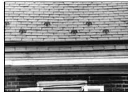
Eave details include snow guards, snow boards, and gutter treatments. Snow guards are generally used in areas where the ice and snow accumulate to avoid dangerous slides from the roof. Photo: Jeffrey S. Levine.
