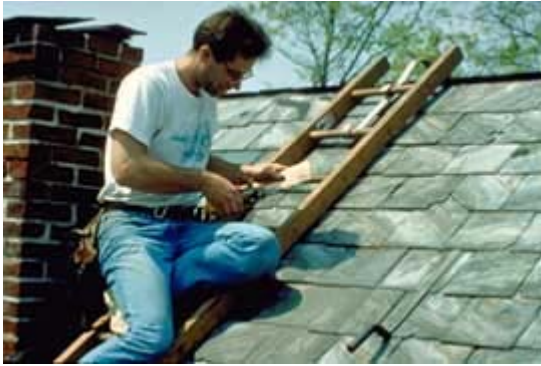
After removing the deteriorated slate and sliding the new slate into place, it is secured with a copper nail. A copper bib (shown here) is formed to protect the newly created nail hole. Finally, a slate hammer is used to push the bib in place over the nail head. Photo: Jeffrey S. Levine.
