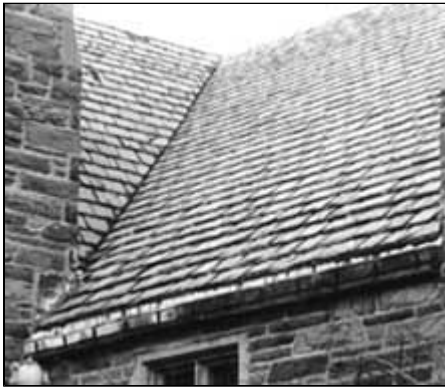
Valleys are formed at the internal angle of two roofing slopes. Flashing is often placed under the slate to increase moisture protection at this vulnerable joint. Photo: Jeffrey S. Levine.
