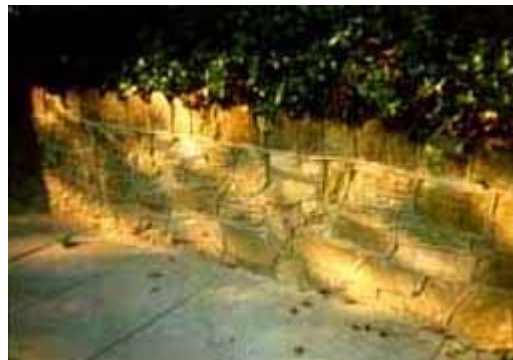
When repairing this stone wall, the mason matched the raised profile of the original tuckpointing. Photo: NPS files.
