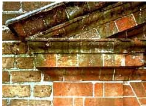
This 18th century pediment and surrounding wall exhibit distinctively different mortar joints. Photo: NPS files.
