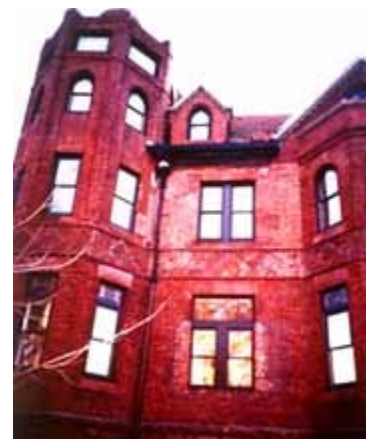
Unskilled repointing has
