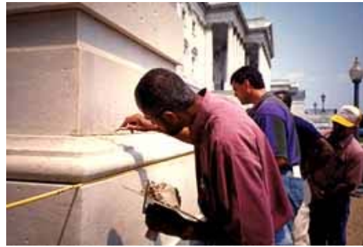
Masons practice using lime putty mortar to repair historic marble. Photo: NPS files.
