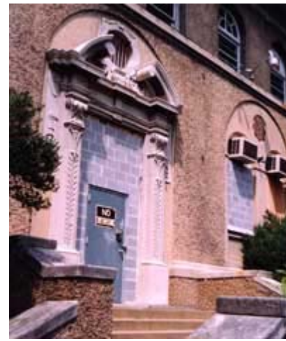
The first floor openings of this historic building have been filled with cinder blocks and the doors, window sash, and frames removed for safe keeping. The security metal door features heavy duty locks. Photo: NPS files.
