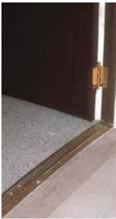
The historic threshold was made accessible with a 1/2" wood bevel. Photo: NPS files.
