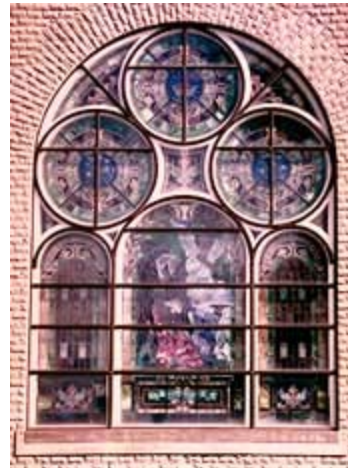
The grid for this protective glazing disregards the configuration of the historic window. The new framing system also causes distracting shadows on the interior. Photo: Neal A. Vogel.
