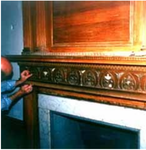
A conservator replaces broken pieces of compo ornamentation on a mantel during a restoration project. Photo: Courtesy, Irving Haynes and Associates.
