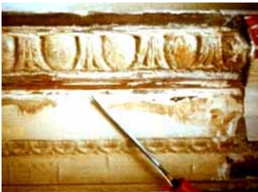
When this historic composition window surround was mistakenly identified as plaster, then treated with a caustic stripper, a section of it was destroyed. Photo: Bryan Blundell.
