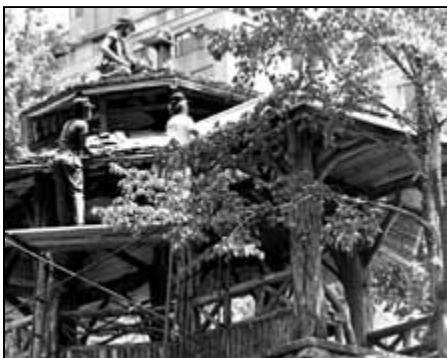
Central Park has developed an in-house historic preservation crew to undertake small projects. A specialized crew has been trained to repair and rebuild rustic furnishings. Photo: Central Park Conservancy.
