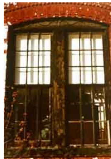
Deteriorating operable windows often contribute to lead dust in a house. In homes
