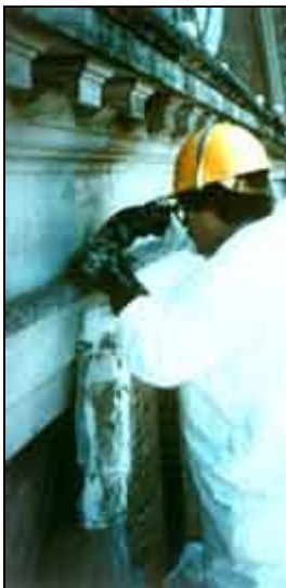
The chemical poultice-type paint remover uses a paper backing that keeps the lead waste contained for proper disposal. Local laws required containment and neutralization of any after-wash water run off. Photo: NPS files.
