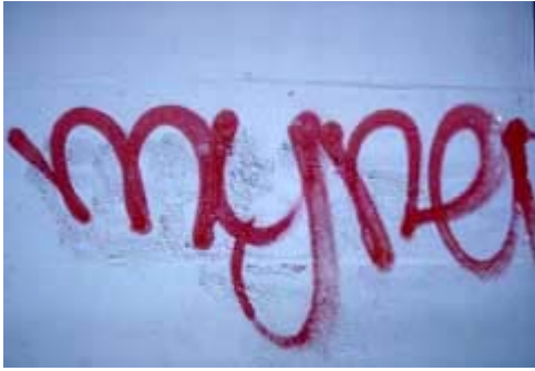
Inappropriate abrasive blasting to remove the graffiti has permanently etched the graffiti into the stone. Photo: NPS files.
