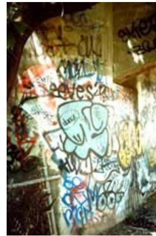
Removing this densely painted graffiti will require several applications of paint remover. Photo: NPS files.
