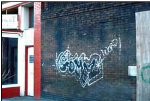
Spray painted graffiti defaces this historic brick building. Photo: NPS files.
