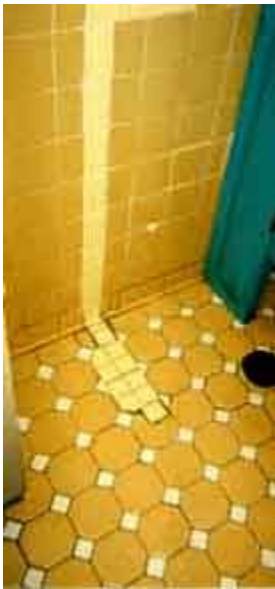
This inappropriate ceramic tile repair is easy to spot. Photo: NPS files.
