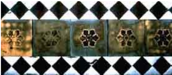
Worn encaustic tiles are still serviceable, but once the design has been lost, the tiles cannot be repaired. They must be replaced in kind, to match. Photo: NPS files.
