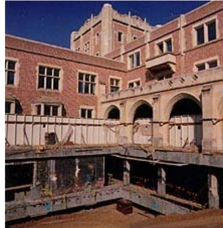
Upon completion, the changes to this ca. 1932 Gothic Revival building to add base isolation at the foundation were not visually apparent. Photo: © Jonathan Farrer
