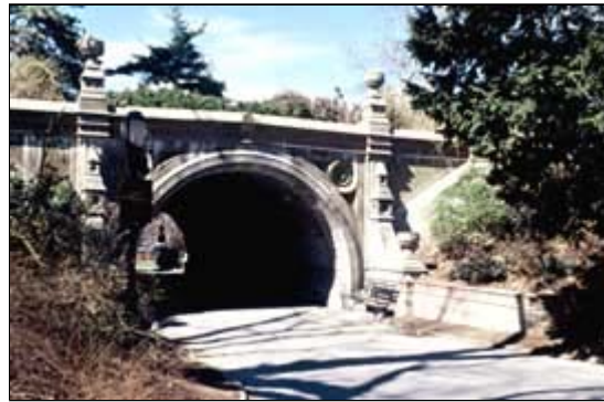
Constructed in 1868 of Beton Coignet, the Cleft Ridge Span in New York City's Prospect Park is one of the earliest extant cast stone structures in the United States. Photo: Richard Pieper.
