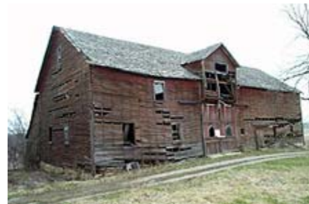
For small or simple projects, the project team may include only one or two specialists while complex projects may involve a large number of investigators and specialists. Evaluation of this barn may primarily involve an historian, an architectural conservator, and a structural engineer. Photo: Wiss Janney Elstner Associates, Inc.
