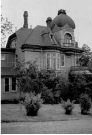
Special problems inherent in the design of an elaborate historic roof can be controlled through regular maintenance. The shape and detailing are essential elements of the building's historic character, and should not be modified, despite the use of alternative surface materials. Photo: NPS files.
