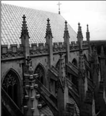
Good design and quality materials for the roof surface, fastenings, and flashing minimize failures. Photo: NPS files.
