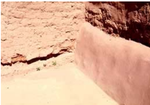
Coving at the base of this adobe wall may have been caused by salts deposited by rising groundwater and/or rainwater splash. Photo: NPS files.
