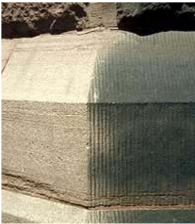
On the left, grit blasting has obliterated the vertical tooling marks from granite, a very dense stone. Photo: NPS files.
