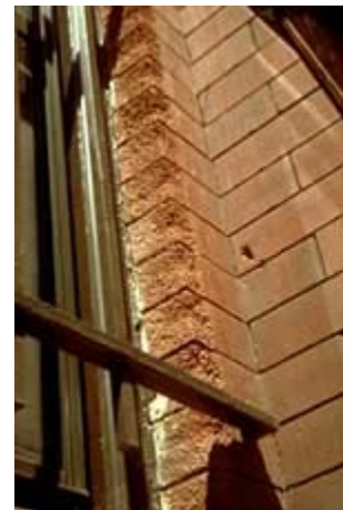
Brick molding next to the window has been severely abraded by sandblasting to remove paint. Photo: NPS files.
