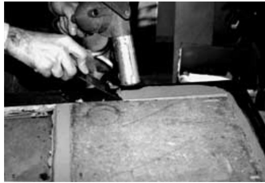
Sash can be removed and repaired in a convenient work area. Paint is being removed from this sash with a hot air gun. Photo: NPS files.
