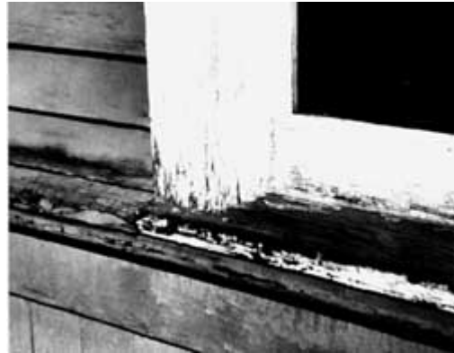
Deterioration of poorly maintained windows usually begins on horizontal surfaces and at joints, where water can collect and saturate the wood. Photo: NPS files.
